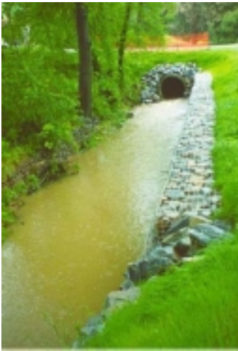
Figure 5. Previous channel armoring of Rocky Branch with gabions. This represents a traditional engineering approach that does not enhance stream aesthetics or habitat, and prevents natural channel restabilization.
