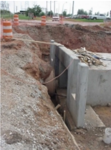
Figure 8. Culvert replacement and installation. Floodplain culvert also added to drain water at bankfull elevation.
