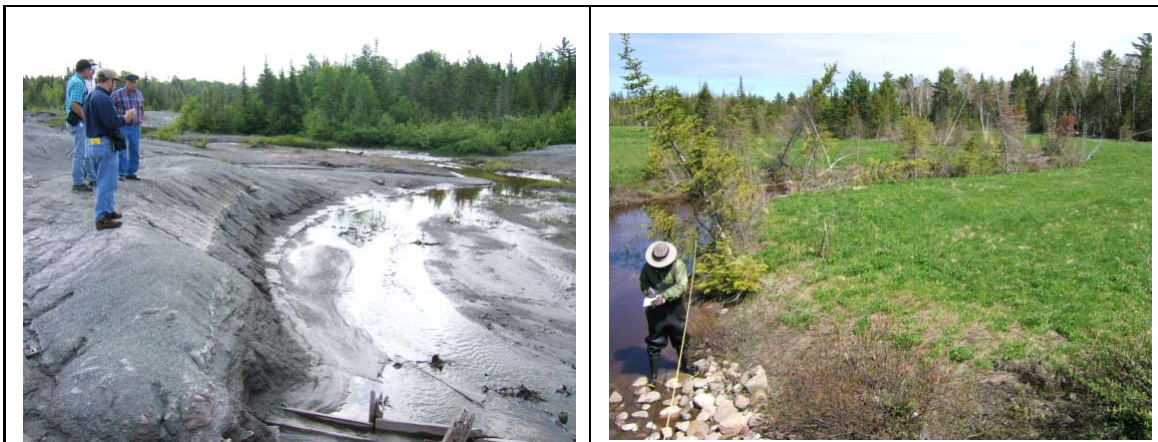
Figure 3. (A) Eagle River at Central 1 before remediation. (B) After remediation (2010), showing the upland vegetation.
