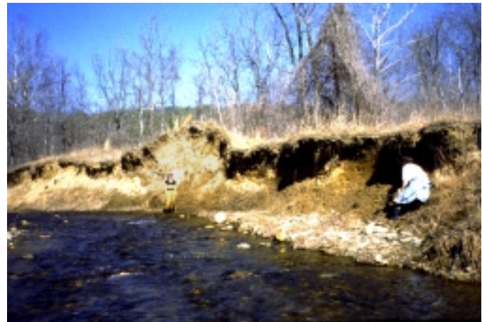
Fig 2: Pre-restoration bank erosion in Reach 4
